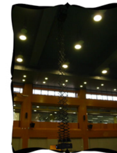
the second level services position
